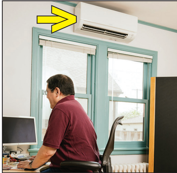
Keep your cool at home even if you don't have duct work. Go with an efficient ductless air source heat pump, instead of a window air conditioner.
