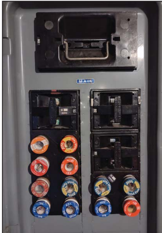
Does blowing the same fuse frequently cause you to blow your fuse personally? That's a sign you need work done on your electrical panel. Upgrade your fuse panel box to circuit breakers for priceless safety reasons and reap a federal tax credit up to $600.
