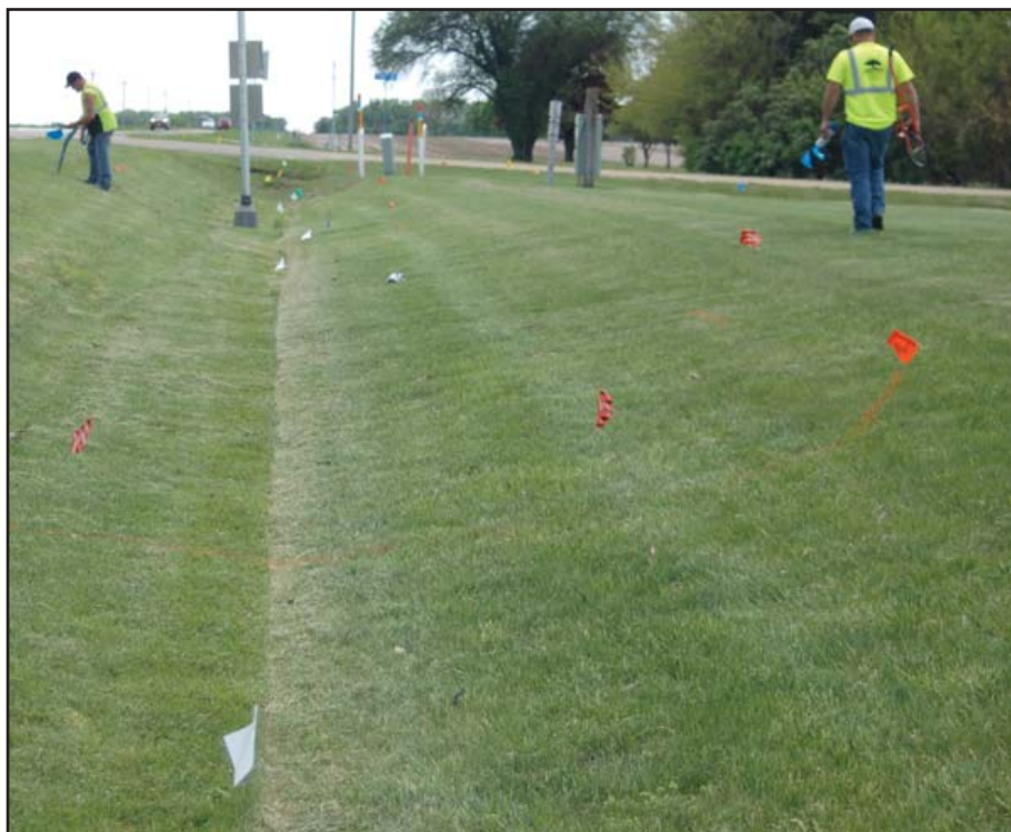
Know what's below. Call Gopher State One Call before you dig so underground locates, like this, can occur marking the underground electric cable, fiber, telephone, gas lines and more.
